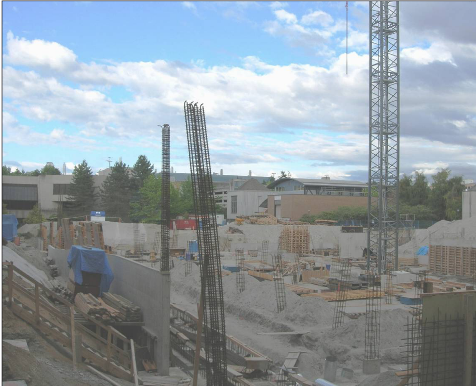
The basement construction of the Beaty Biodiversity Centre, where the UBC biological collections will be housed
